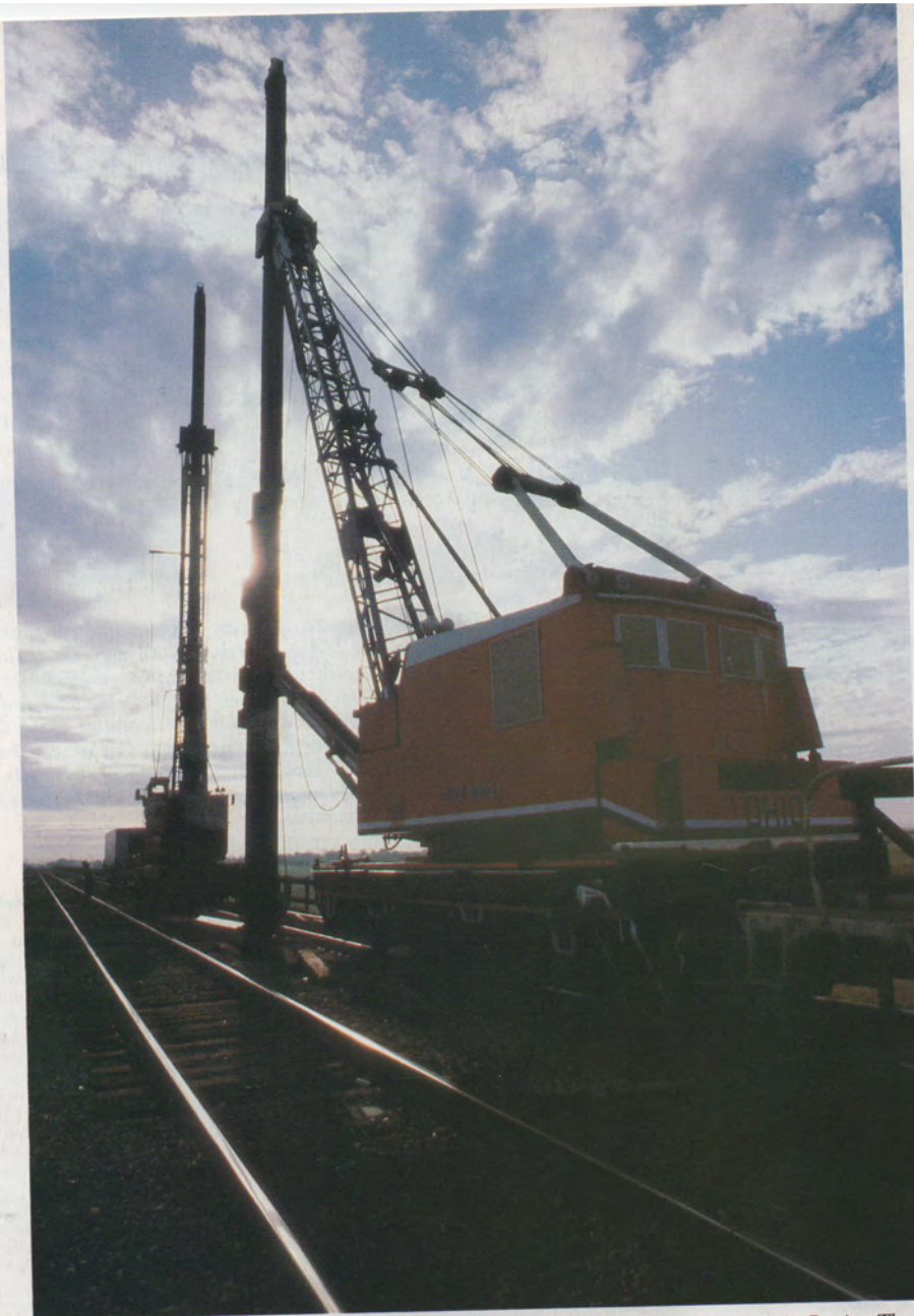
Ninety-foot tall steel beams replace timber pilings in the trestles over the Yolo Basin. The trestles, over the flood way of the Sacramento River, are on our main line between Sacramento and Davis, Calif. They form one of the longest—8,600 feet—series of trestles in the system. See page 18 for the story on this important renewal project.
