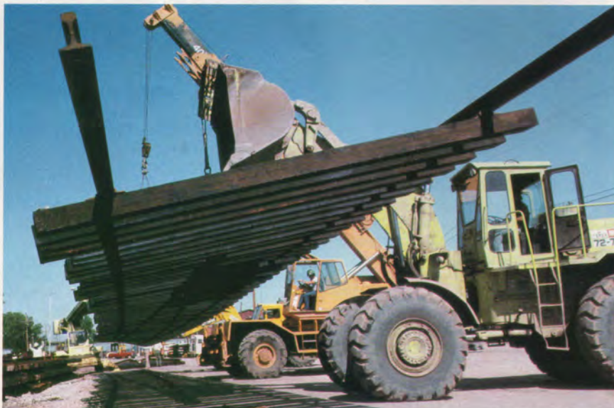
Prefabricated track panels speed up railroad construction projects. This panel is being placed in one of Armourdale's four receiving/departing tracks.
