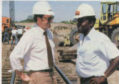
Project Manager Mike Christensen (left) and District MofW Manager L. J. Fletcher are in charge of Armourdale's rehabilitation.
