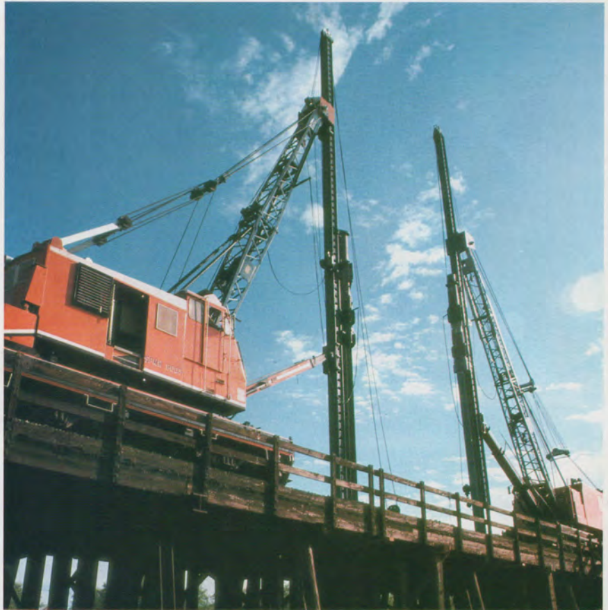
These locomotive cranes, with Paul DeWitt or Larry Blevins at the controls, can lift, lower, position and drive 90-foot steel beams weighing 6,570 pounds.
