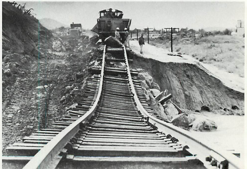
A bridge at Moorpark, between Oxnard and Los Angeles, suffered damage by the heavy runoff from the rains.
