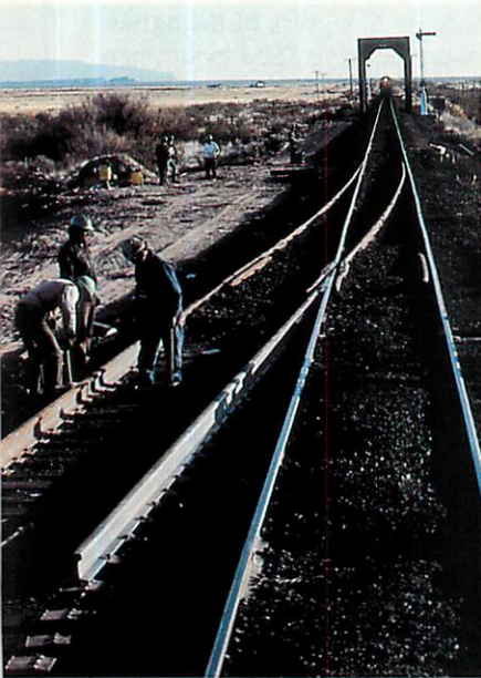
A switch is installed as part of the siding extension work at Three Rivers.
