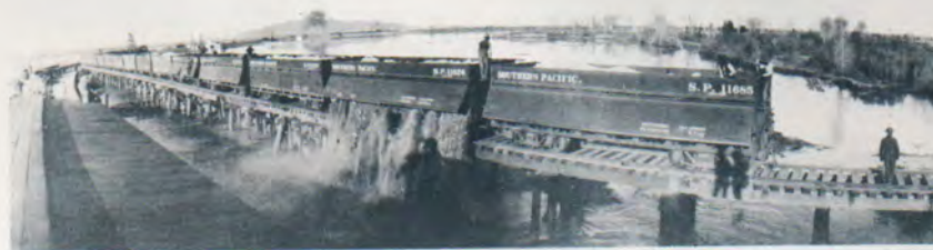
The Colorado River overflowed in 1905-07, creating the Salton Sea and threatening to inundate California's Imperial Valley. After a long battle, SP forces sealed the break at a cost of about $3 million.
